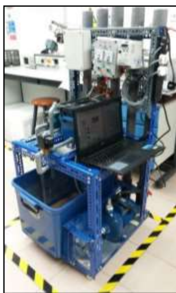
Figure 3: Aluminum Staging Water Filter (ASWF) Plant
