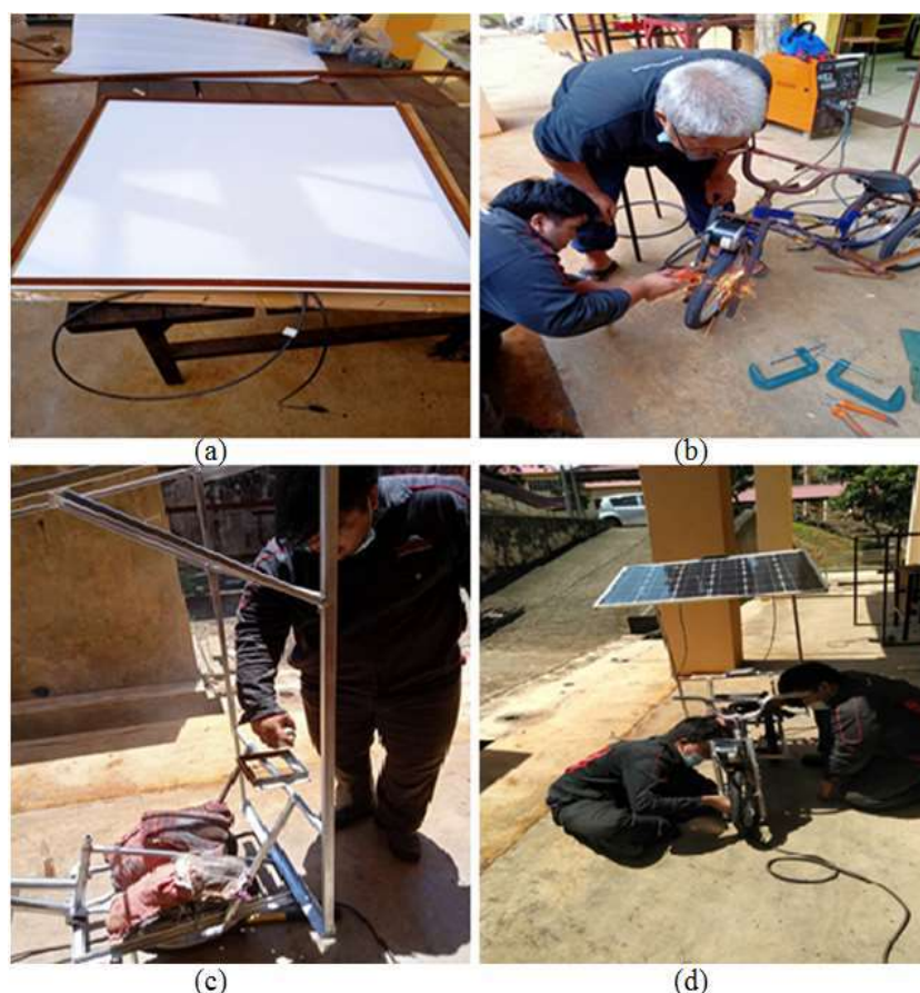
Figure 4. (a) Solar panel mounting (b) Weld joint on frame parts (c) Spray painting on frames (d) Installing
