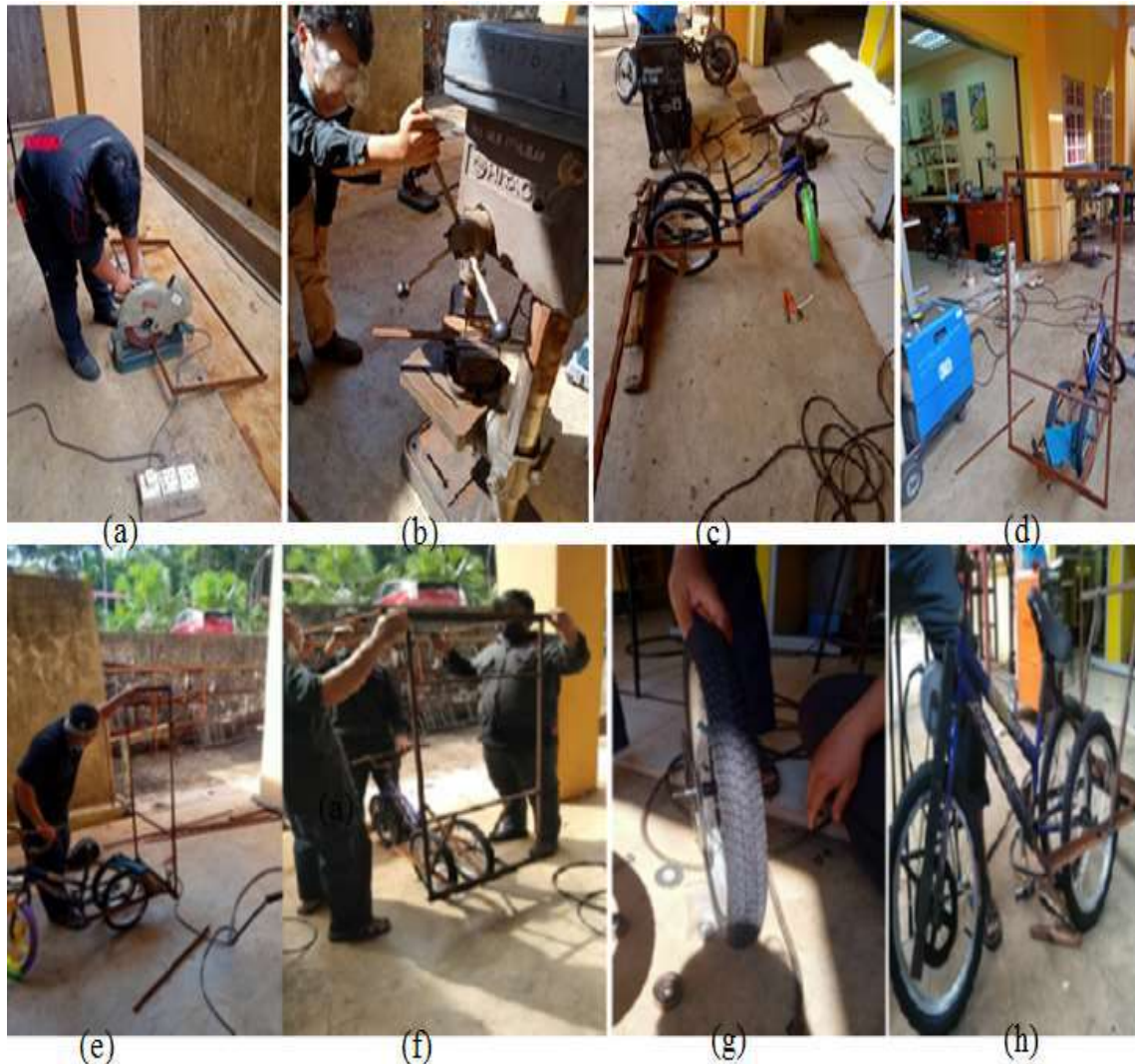
Figure 3. (a) MS cutting for frame parts. (b) Drilling for brackets and mountings. (c) Arrangement of rear wheel frame. (d) Vertical frame for solar mounting. (e) Alignment of vertical frame. (f) Preparation for top solar panel mounting frame. (g) Arrangement of chain drive on front wheel for power transmission. (h) Alignment of power transmission system.
